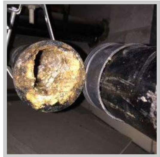
Photo provided by UC Berkeley Facility Services: Sanitary sewer pipe cross-section with build-up of FOG; the blockage narrows the pipe and restricts the volume of water that can flow through the pipe.
