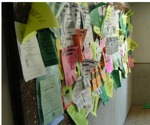
An Unacceptable bulletin board. Materials are not secured on all corners and there is too much accumulation of combustible material due to layering of flyer's.
