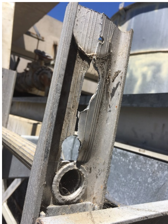
Photo 1 - The Sheared Metal Ladder
